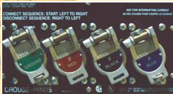
Quick connect couplers are used on both the control house and main trailer.
