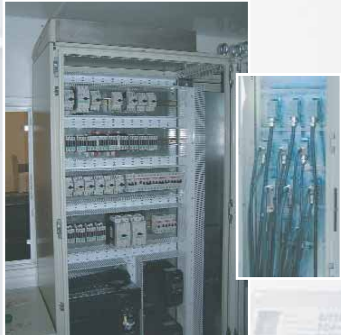
The variable frequency drives for all the unit's motors are housed within the control house and cooled by a dedicated air-conditioner. The image at the right shows the quick disconnect panel on the outside wall of the control house.
